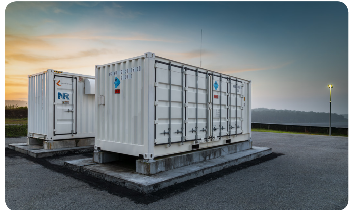
250 kWdc/1.45 MWh-dc NaS ® battery energy storage system which is integrated with Leader Energy's 20 MWac Grid Connected PV System (GCPV) solar plant located in LSE II, Sungai Petani, Kedah
